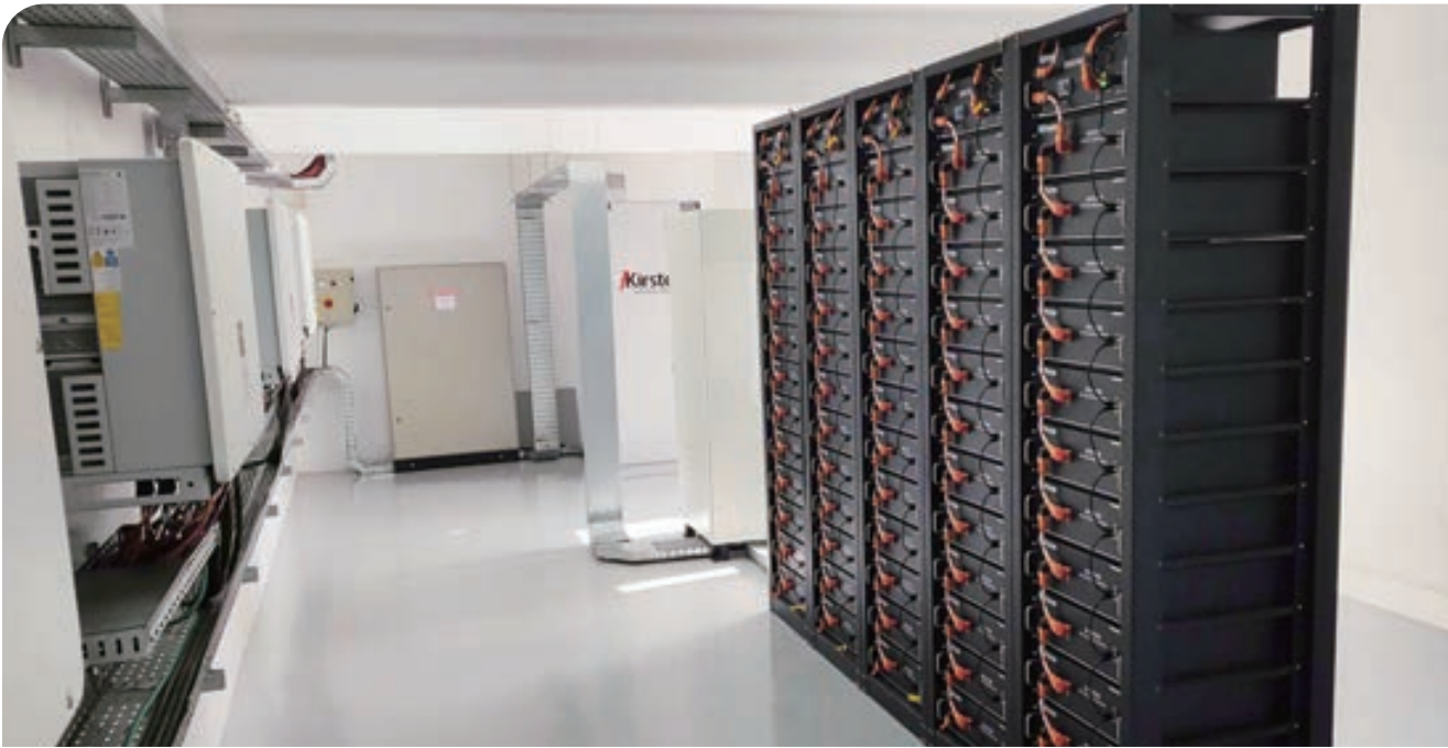
• Brazil PowerRack HV4
